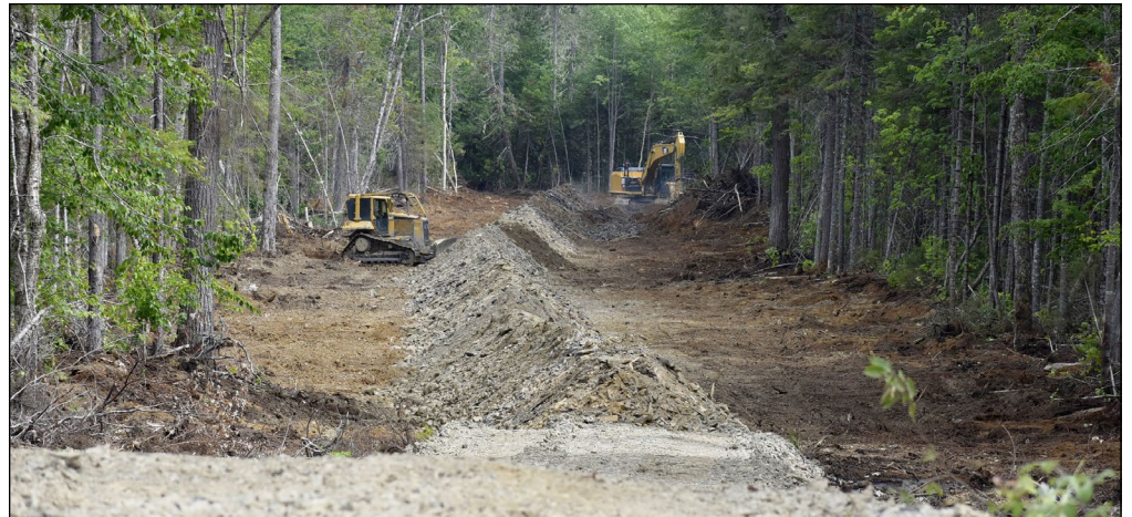
With the summer season now in full swing, a new section of forest road is being constructed and prepared for use.
